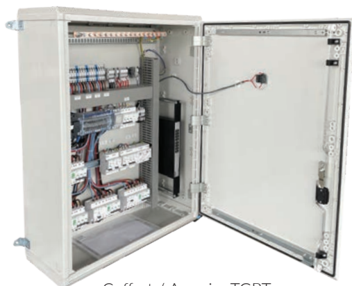
Coffret / Armoire TGBT
